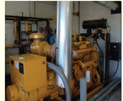
Figure 2. Internal Combustion Engine and Generator.
